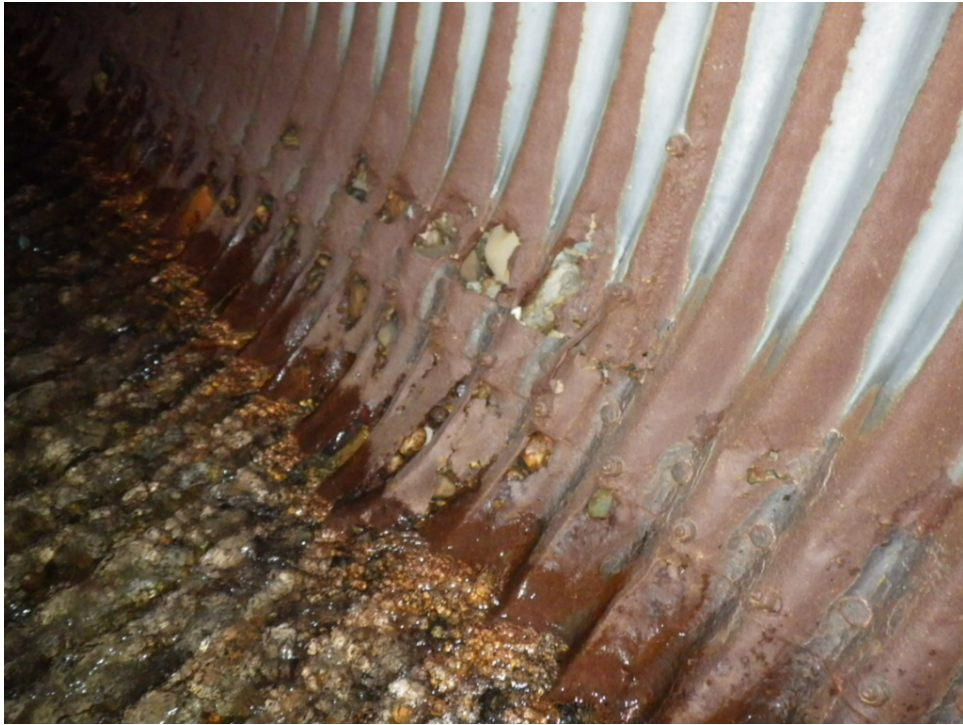
Picture 5: Holes Forming on Invert
